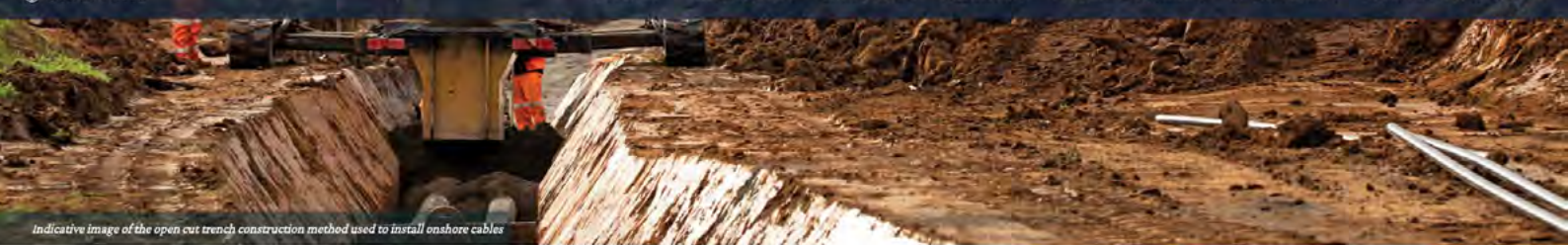
Indicative image of the open cut trench construction method used to install onshore cables
